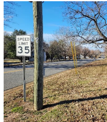
Above ground utilities on 34th Street
